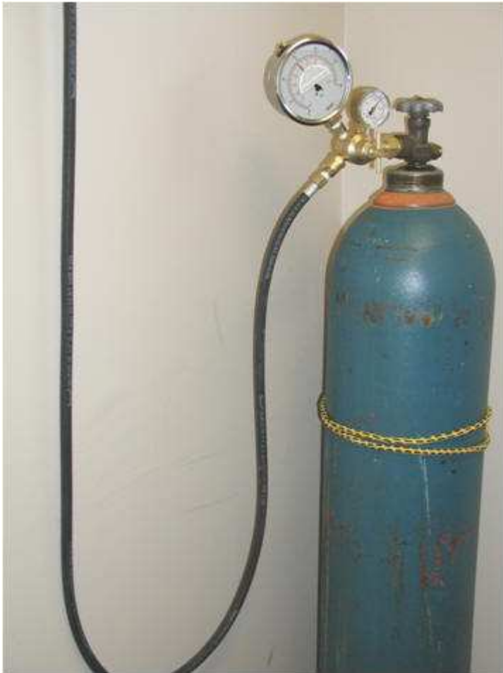
Nitrogen Tank with Pressure Gauges and Regulator
